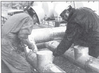
Workers from Aadri Ltd. inspect a section of their above-ground heat-recycling pipe network.
